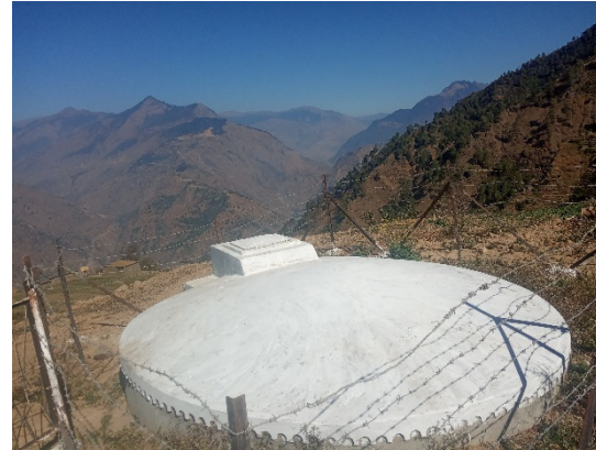
Picture 40: Water Distribution Tank
