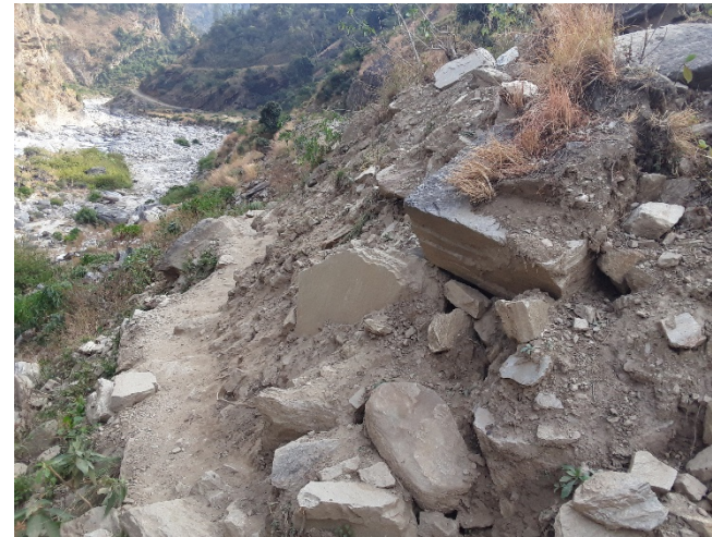
Picture 4: Narrow width due to rock slide
